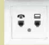
MBR819 : Telephone Socket & Computer data socket
